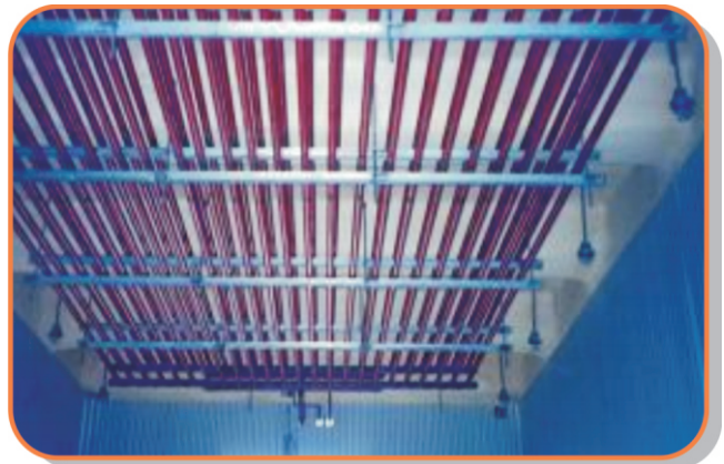
B. STEEL COOLING COIL
